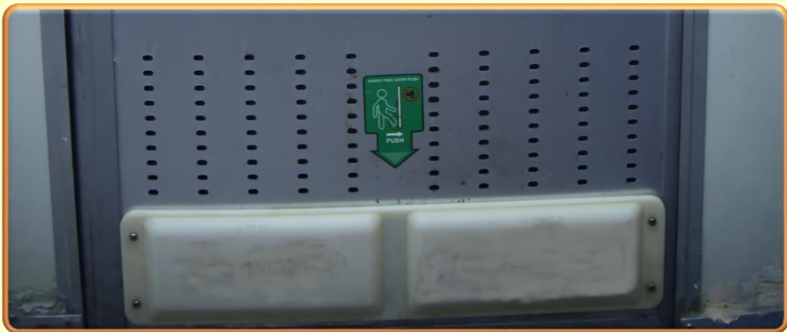
Foot operated Lavatory door (outside)
